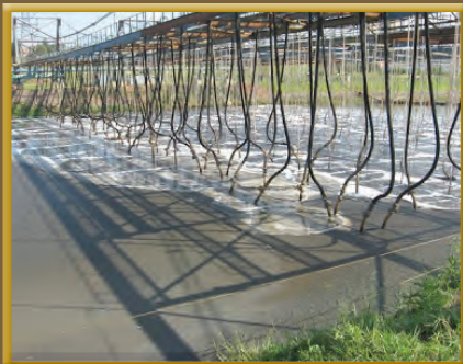
An in-river application in Brazil, which can also be seen in the above aerial photo
